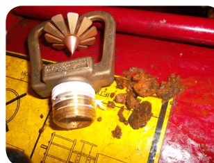
Corrosion removed from deluge nozzle
