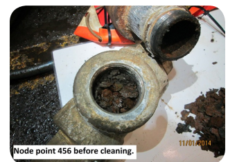
Corrosion Product in deluge pipe
