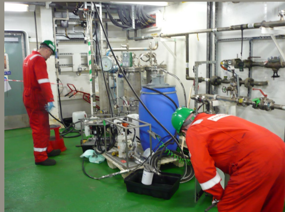
2 x Air Driven Pumps, Break Tank & 2 x Returns Filters
